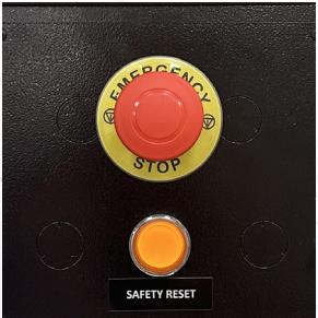
Emergency Stop Pushbutton
